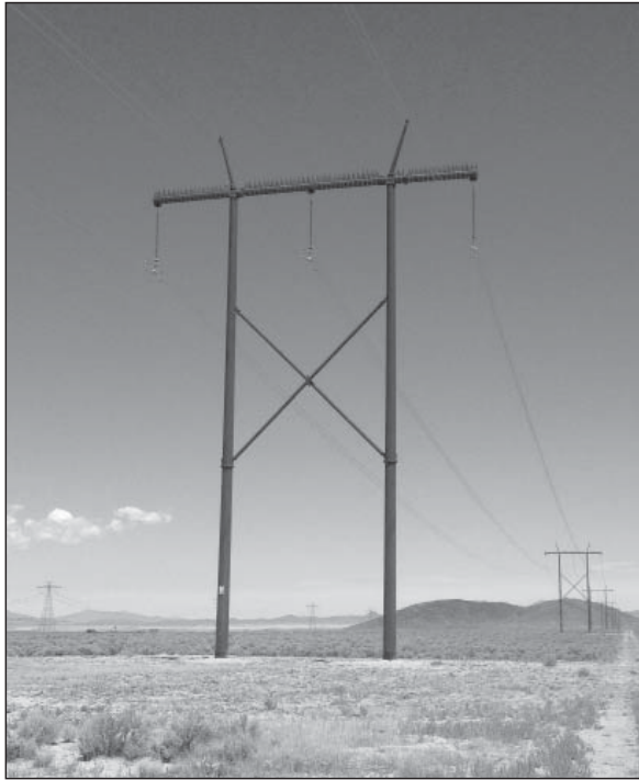
Figure 2. Typical H-frame tower with installed perch deterrents which comprised the Sigurd-Red Butte 345-kV transmission line, constructed fall 2014. (Photo by E. Hansen)
