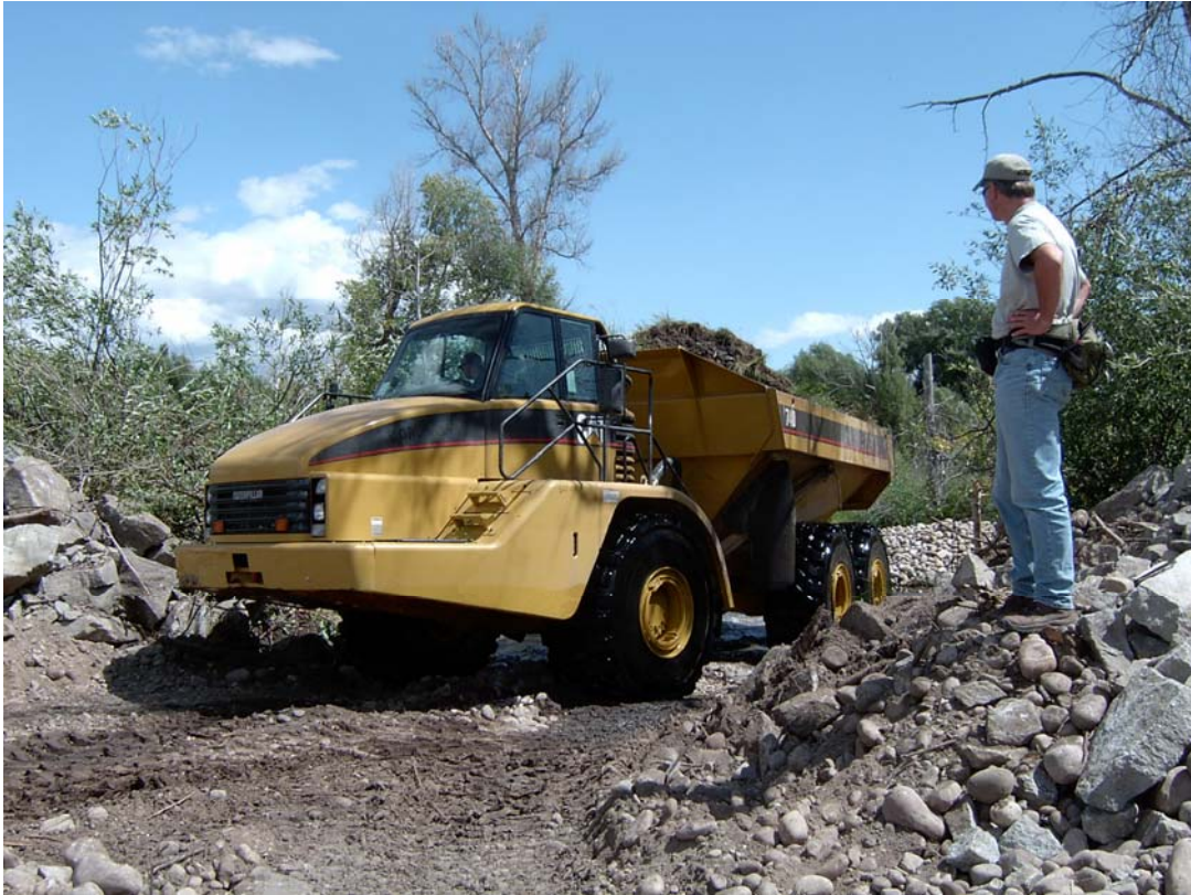
Figure 3-4. This truck, common amongst equipment used in construction of the PRRP, is shown transporting excavated material via the bed of the reconfigured channel that is under construction.
