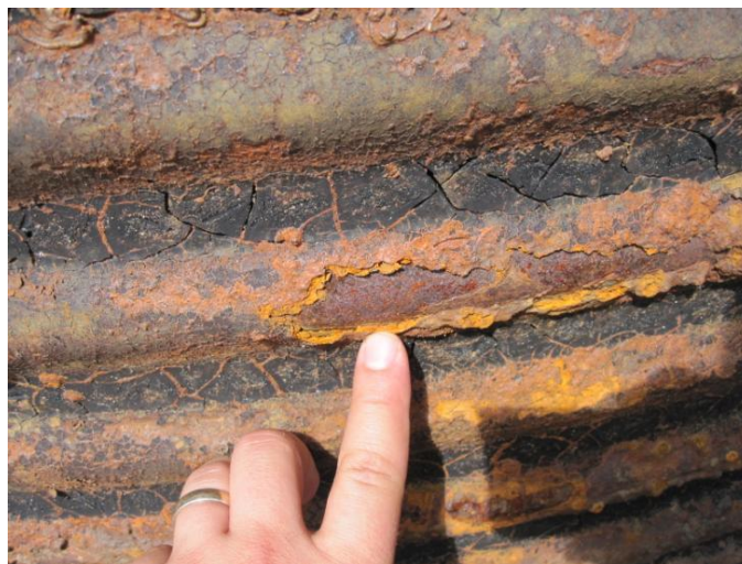
Figure 2. Half-pipe riser weir's sheet metal skin experiencing pitting corrosion after one use cycle with protective asphaltic coating.
