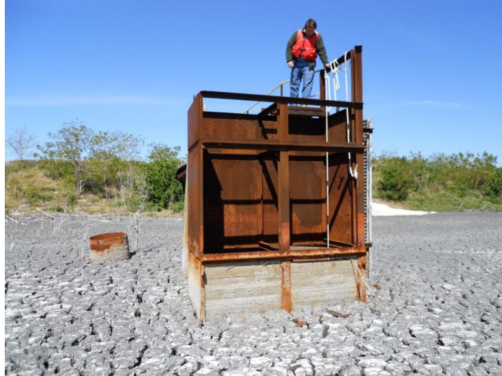
Figure 1. Box riser weir crevice corrosion at water-air interface after one use cycle.
