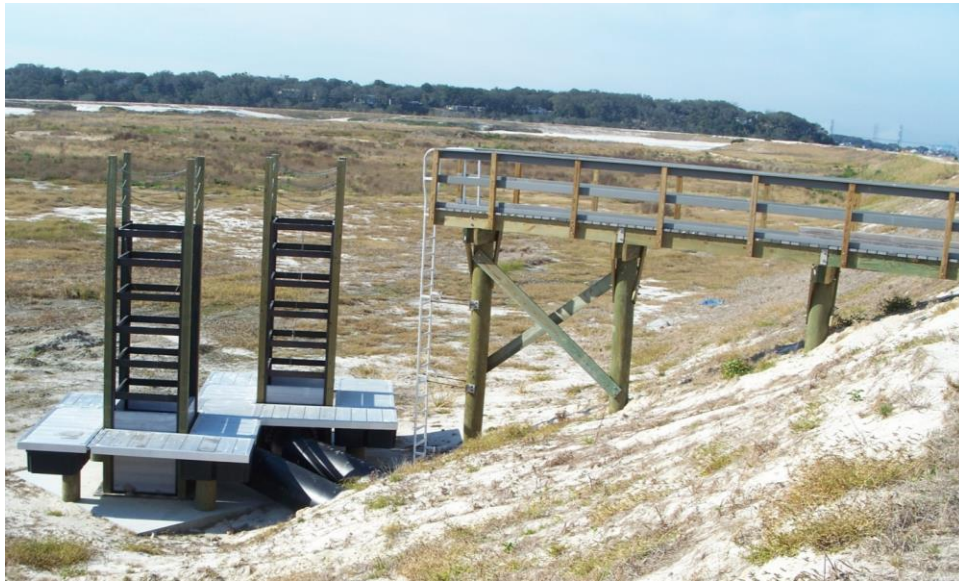
Figure 4. Set of 4.9 m (16 ft) tall 1.2X1.2 m (4x4 ft) Box Riser Weirs with floating dock access, Buck Island, Jacksonville, Florida. (Maglio et al. 2014).
