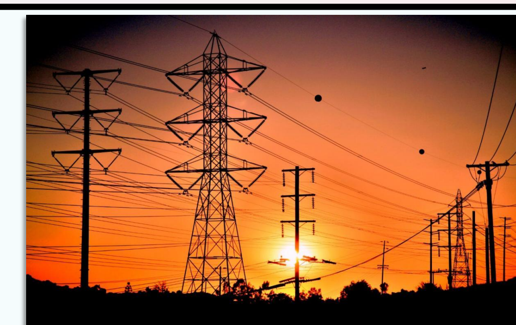
Figure 11. High voltage power transmission lines. Photo by Dennis Richardson
