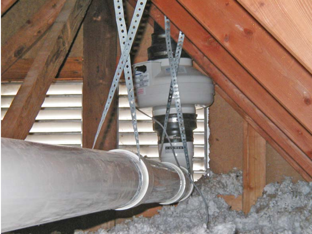
Figure 6. Interior VRS fan installed in a residence near Hill AFB.
