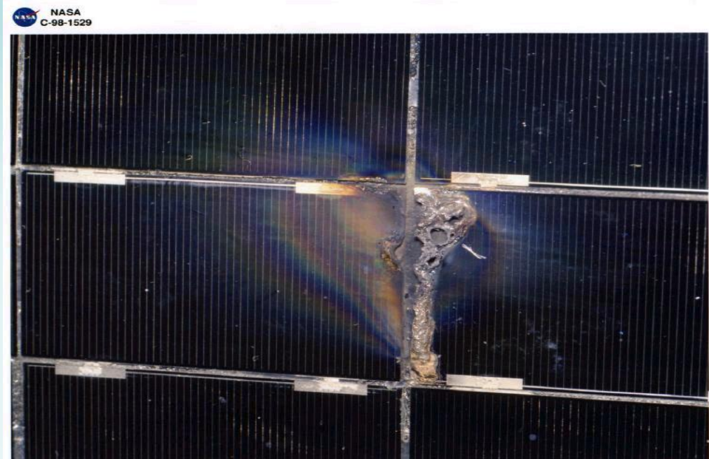
Solar panel damaged by localized charging event
