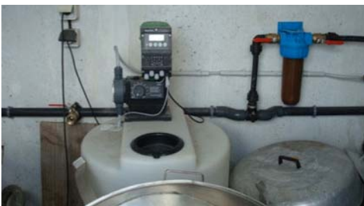
Figure 7. Water treatment. (LDS Church, 2010)
