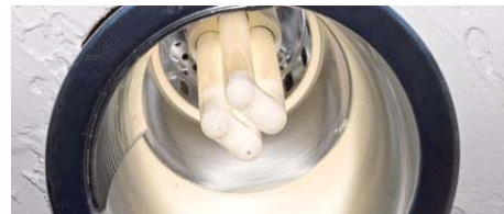
Figure 19. High efficiency lighting. (LDS Church, 2010)
