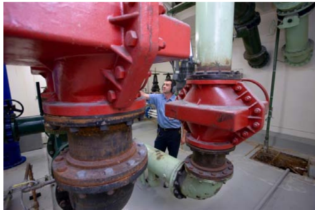
Figure 16. Geothermal pumps under LDS Church Office Building. (LDS Church, 2010)
