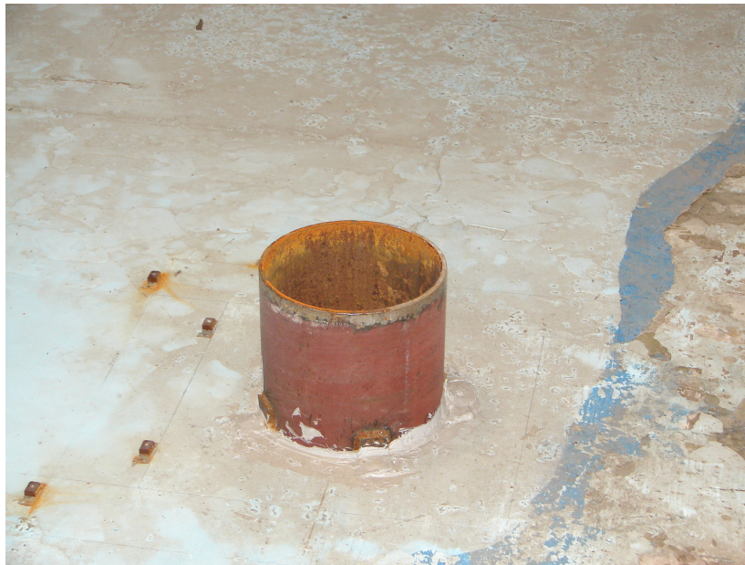
Figure 4. 12" diameter intake pipe.
