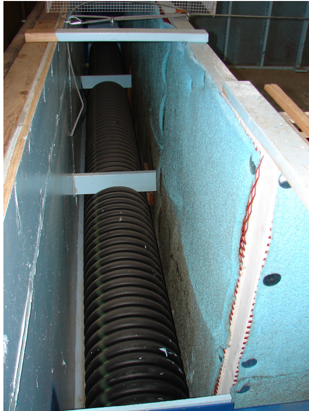
Figure 5. Diffuser and distribution piping.
