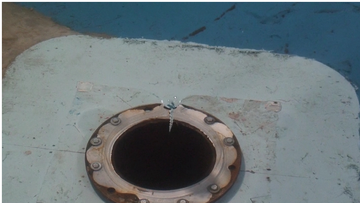
Figure 2. SNWA Intake #2 without debris cage.
