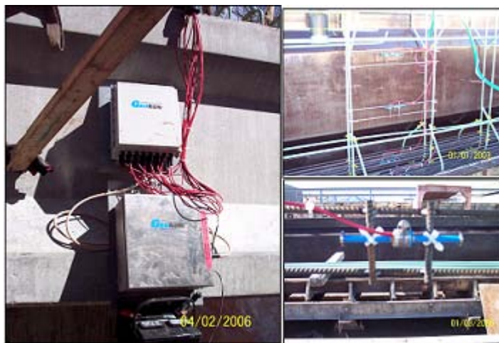
Figure 2.3. Bridge instrumentation equipment.
