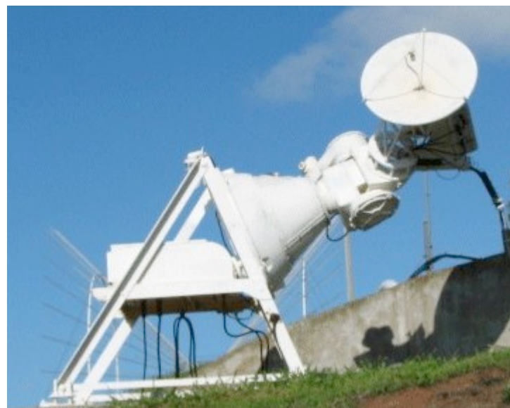
Figure 3.5: 3-ft parabolic dish antenna at Palehua Solar Observatory is used to monitor 15,400 MHz. The antenna is mounted on top of the tracking mechanism.
