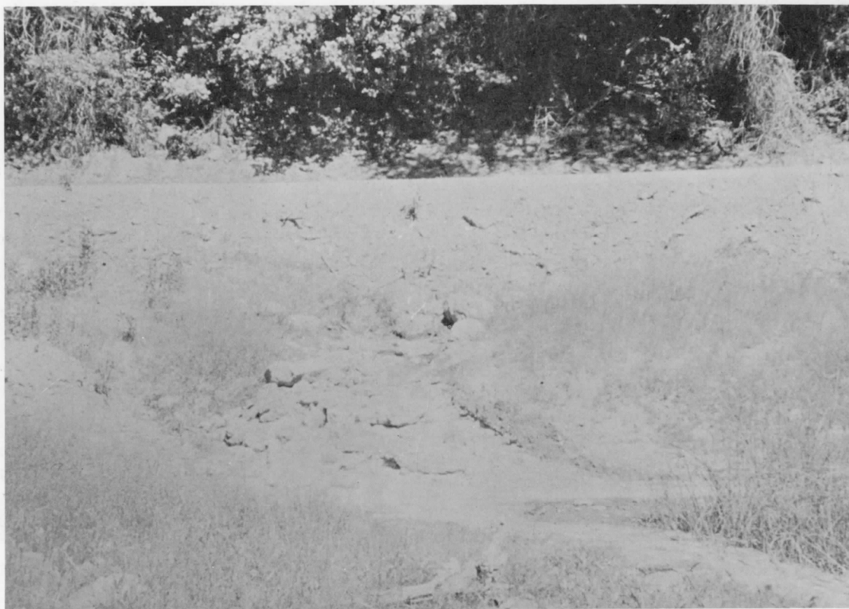
Fig. 23. Diamond Fork Warm Spring at the base of the road fill.
