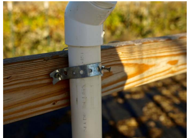
Figure 8. Plumber's strap can be used to hold the purlin to the sidewall. A screw will hold the purlin up until the covering is in place. Then the screw can be removed and the anchor ties can be used to keep the cover taut.
