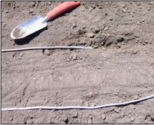
Image 2. Buried electric heating cables.
