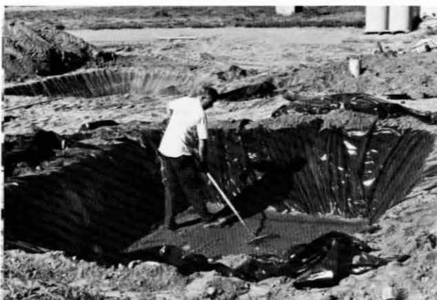
Fig. 8. Construction of experimental alkali bee nesting sites. Plastic in place, protective soil layer being installed. (H. W. Potter)
