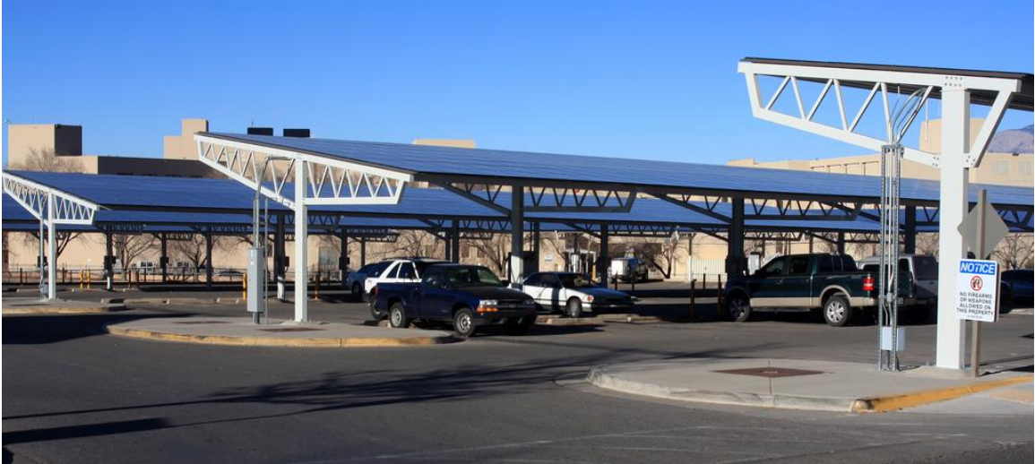
Figure 9. Solar parking lot canopies at the VA Medical Complex in Albuquerque, NM. By J.N. Stuart, 2011, retrieved from https://www.flickr.com/photos/stuartwildlife/with/8402076067 Reprinted with permission.
