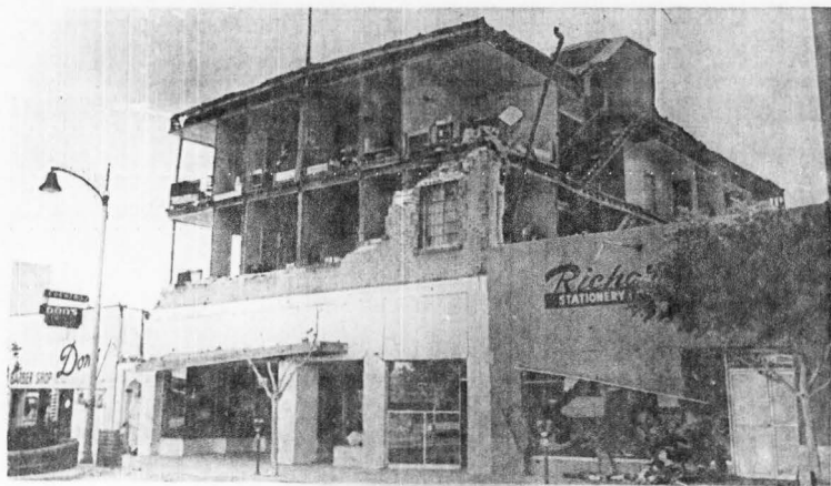
Figure 3-6. Total collapse of brick masonry wall surrounding three-story wood frame building (after Lew, Leyendecker and Dikkers, 1971).
