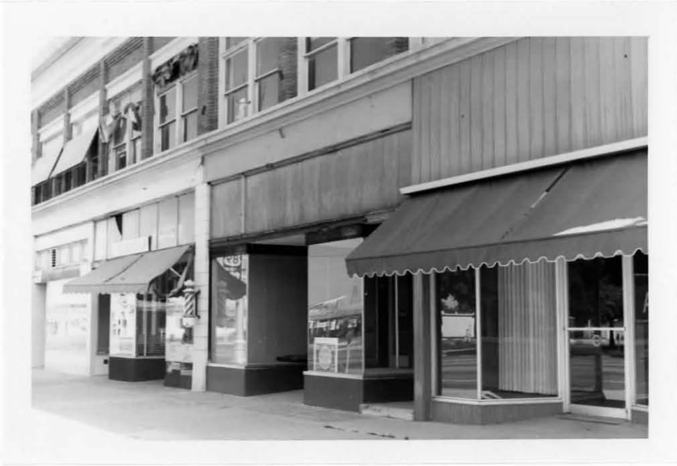
Figure 31. Shabby appearance of building
