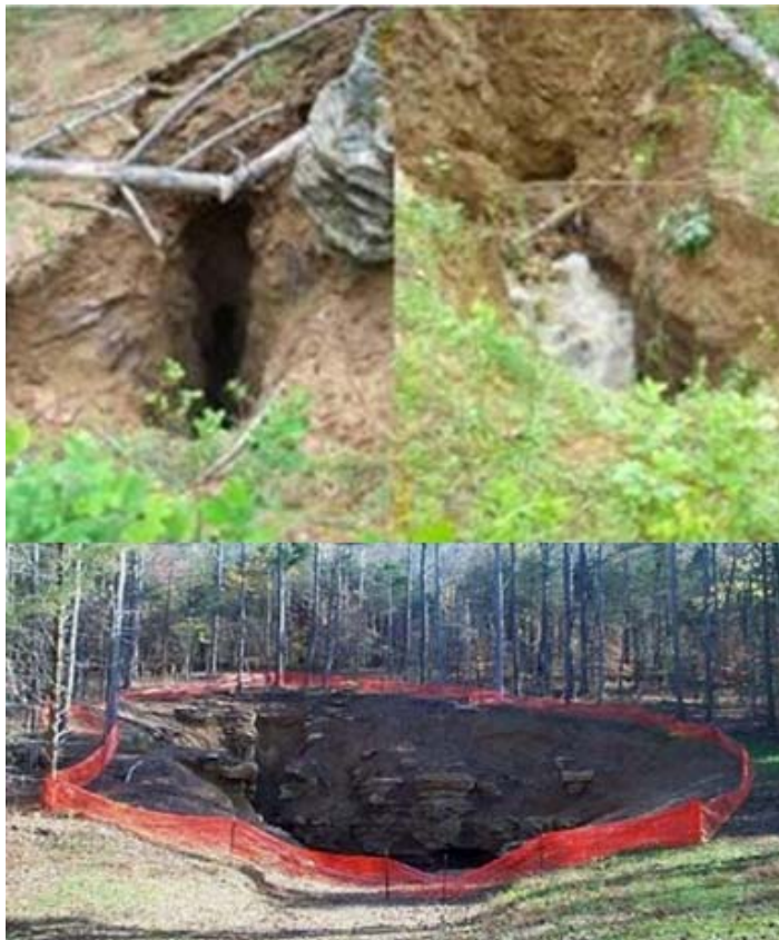
Figure 7. Left rim sinkholes at Center Hill Dam (Brimm 2010)
