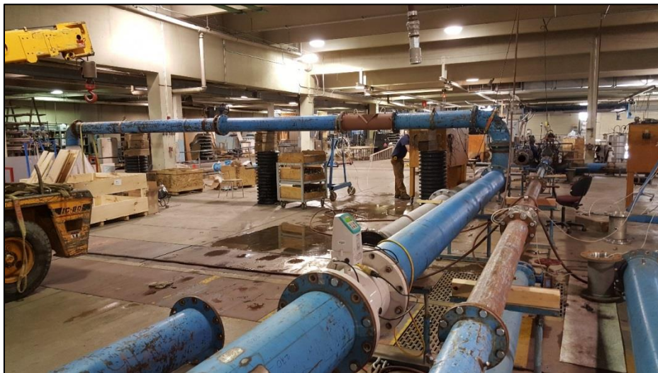
Figure 3: Laboratory Flowmeter Installation
