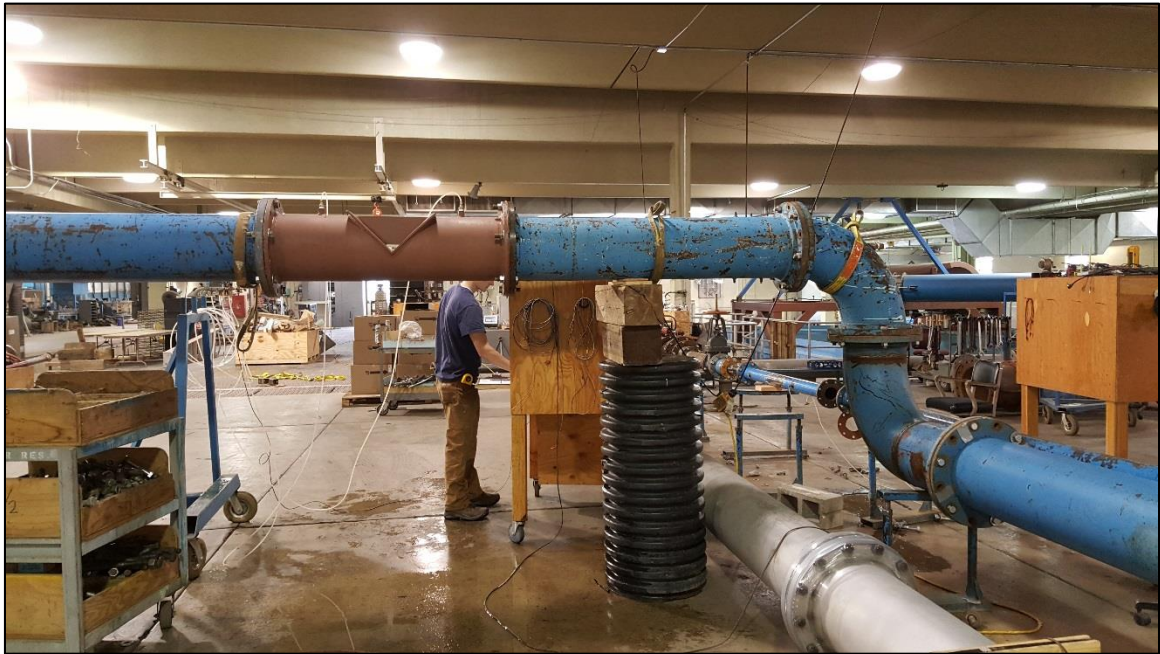
Figure 5: Wedge Flowmeter Five Diameters Downstream to DEOP in the Vertical Position
