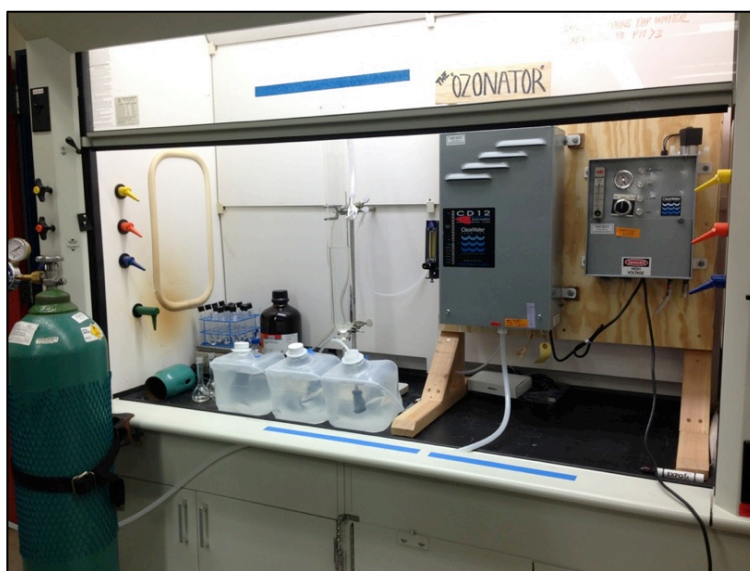
Figure 12. Clear Water Inc. ozone generator.
