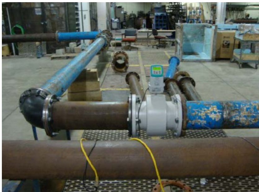
Figure 4. Phase I 3D Pipe Test Setup (flow left to right)
