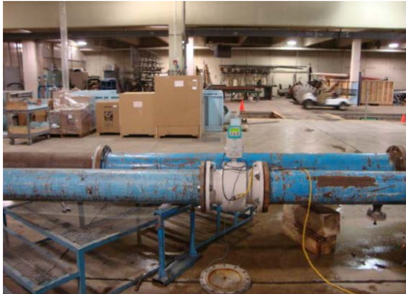
Figure 3. Phase I Straight Pipe Test Setup (flow left to right)
