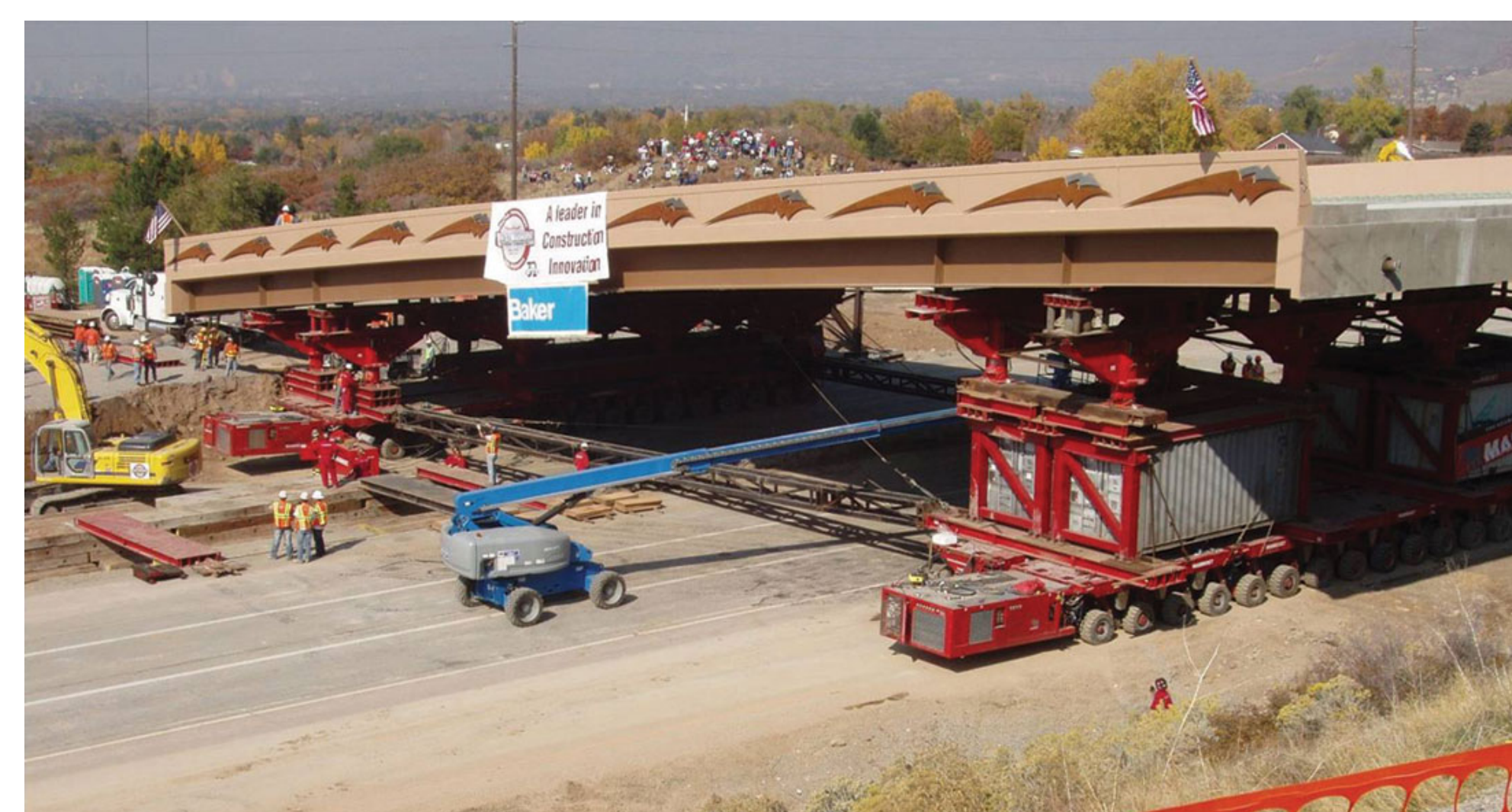
SPMT's in use during the construction of Utah's I-215 / 4500 South Bridge. (Federal Highway Administration.)
