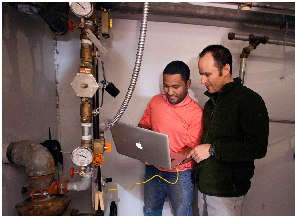
Utah State University Assistant Professor of Civil and Environmental Engineering Jeff Horsburgh, right, and student Miguel Leonardo Feliz work to configure a new smart water meter at a campus dormitory building.
