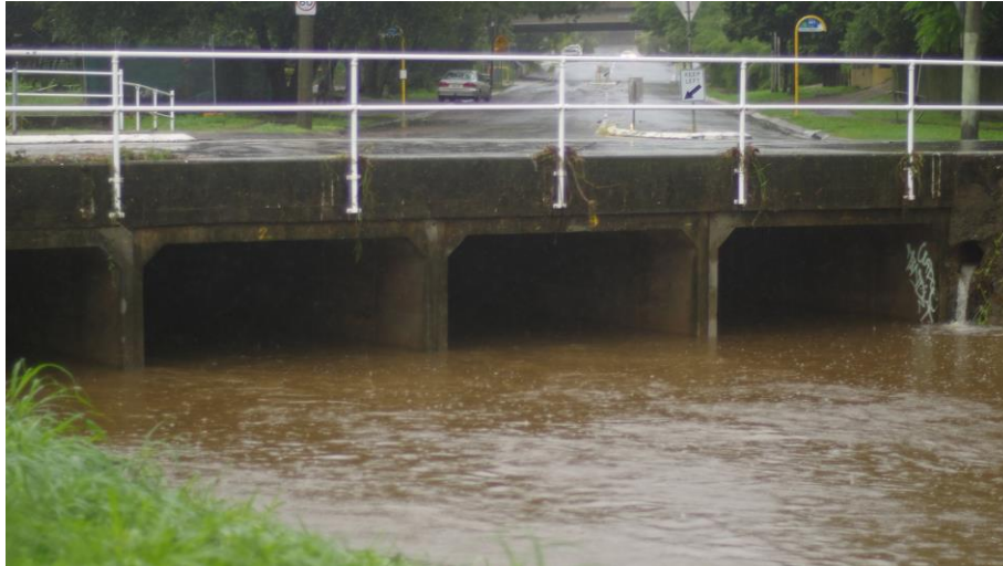
Figure 1. Standard box culvert along Whitton Creek, below Kale St, Chapel Hill QLD (Australia) on 30 March 2017 at the end of a major rainstorm
