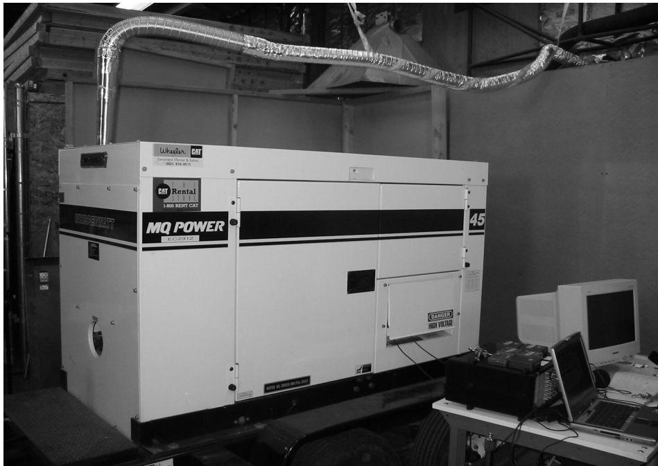
Figure 1 Apparatus to be controlled: 45KVA (36kW) diesel generator
