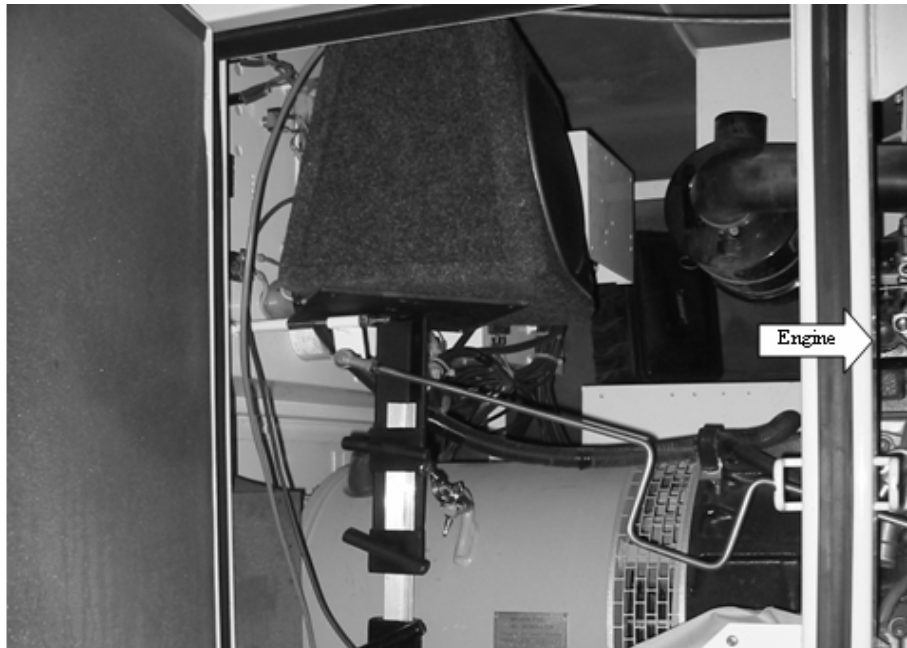
Figure 3 Control source (8" SUB) mounted inside generator enclosure
