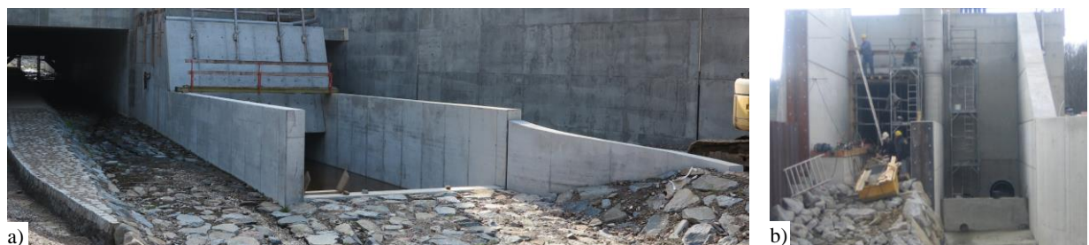
Figure 2. Separation of the ecological culvert and the operation outlet: a) FRB Niederpöbel, Saxony (recently under construction); b) FRB Rennersdorf, Saxony (construction period 2006-2010).
