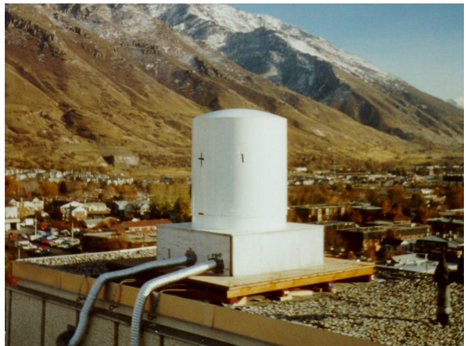
Fig. 2. Receiver of the SeaWinds Calibration Ground Station. Tubes pump cool air into the radome and protect sensitive cables connected to computers below.
