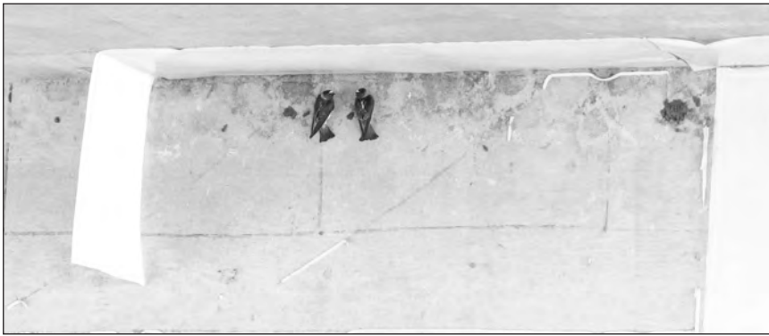
Figure 10. PTFE sheets detaching from the concrete bridge surface and cliff swallows building nests.
