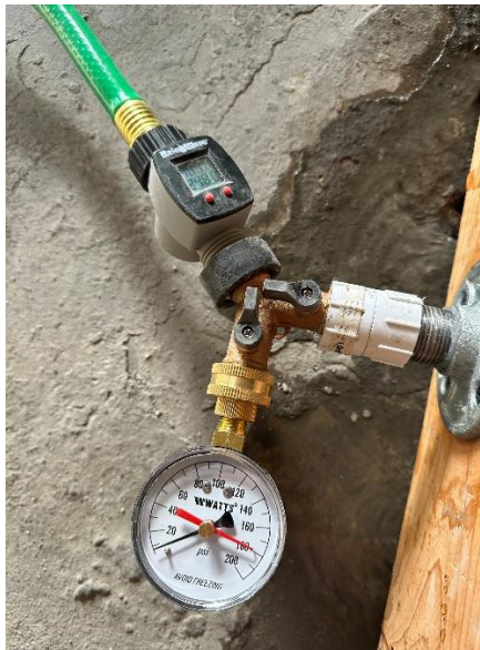
Figure 3-10: Pressure gauge and flow meter attached to hose
