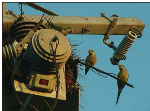
Parakeets nesting in power transformer.
