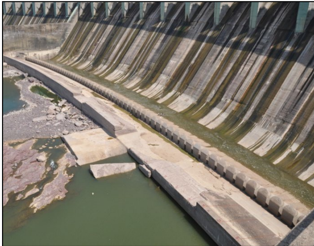
Photo 1. Damage to bucket portion of spillway
