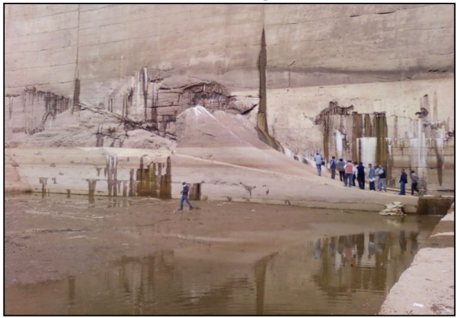
Photo 4. Exposed reinforcement of teeth
