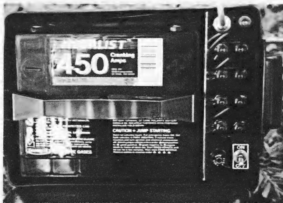
b) Battery Box, inside view
