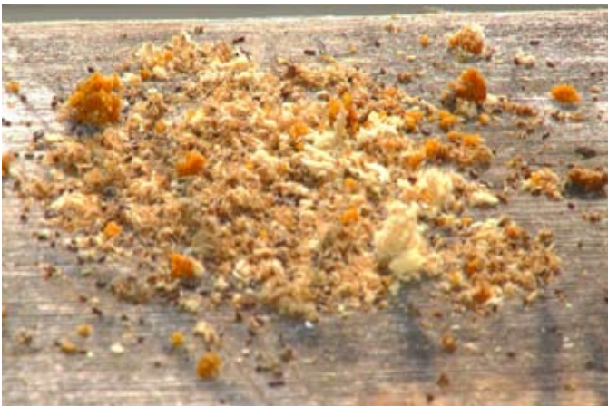
Fig. 6. Carpenter bee castings, including excavated wood dust and excrement. 4
