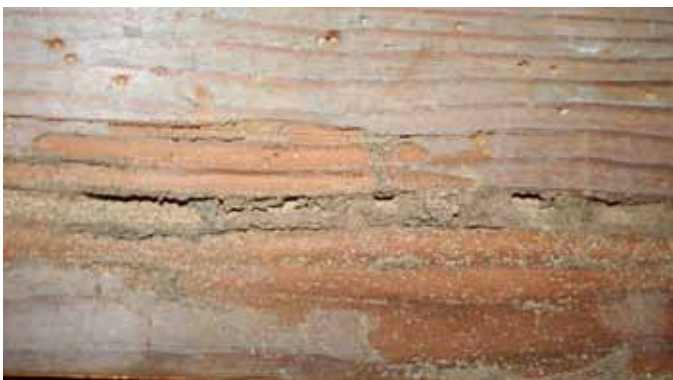
Fig. 8. Subterranean termites often feed along the spring wood and leave behind frass. 7
