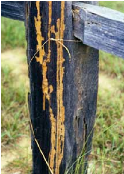
Fig. 7. Eastern subterranean termite mud tubes on a post. 6
