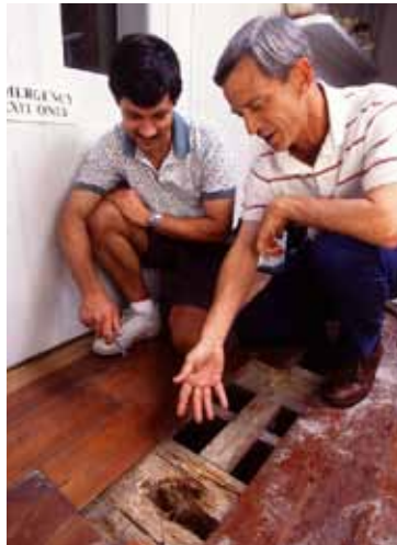
Fig. 10. Subterranean termites can shred solid wood beams. 4
