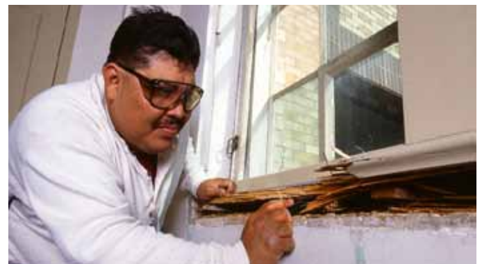
Fig. 9. Heavy subterranean termite feeding damage can cause paint to blister. 4
