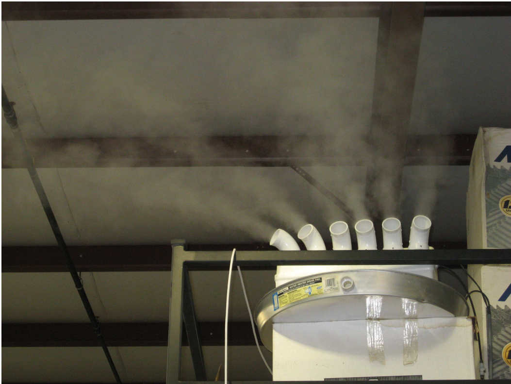
Fig. 3-4. A Humidifirst MP15 ultrasonic humidifier is used to maintain the humidity at levels needed for efficient production.
