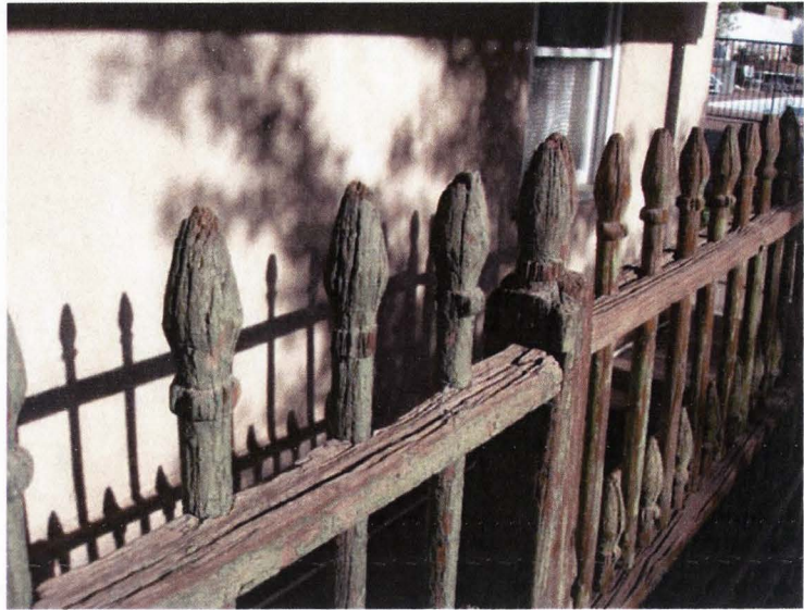
Fig. 26 Original lathed picket gate on display at the Greene Gate Village Bed and Breakfast. The green paint is historically significant as well (2007).
