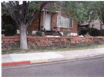
An existing dry stack sandstone and basalt rock wall more than 70 years old. This wall is less than 3' tall.
