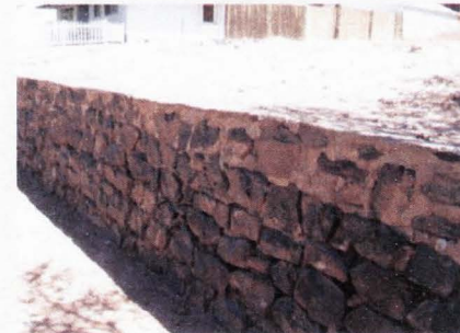
A portion of the same basalt rock wall with characteristics of both dry stack and mortared joints.
