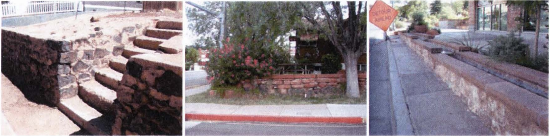
Fig. 21 The image on the left shows a basalt rock retaining wall. The middle image shows a wall that combines both basalt and sandstone that is over eighty years old. The image on the right shows current wall construction practices that are inconsistent with the historic character.
