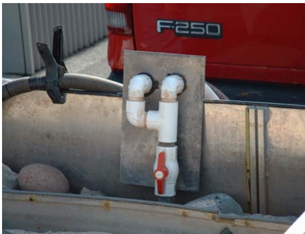
Picture E: Valve B
