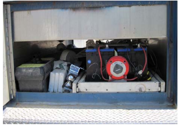
Picture H: Batteries
