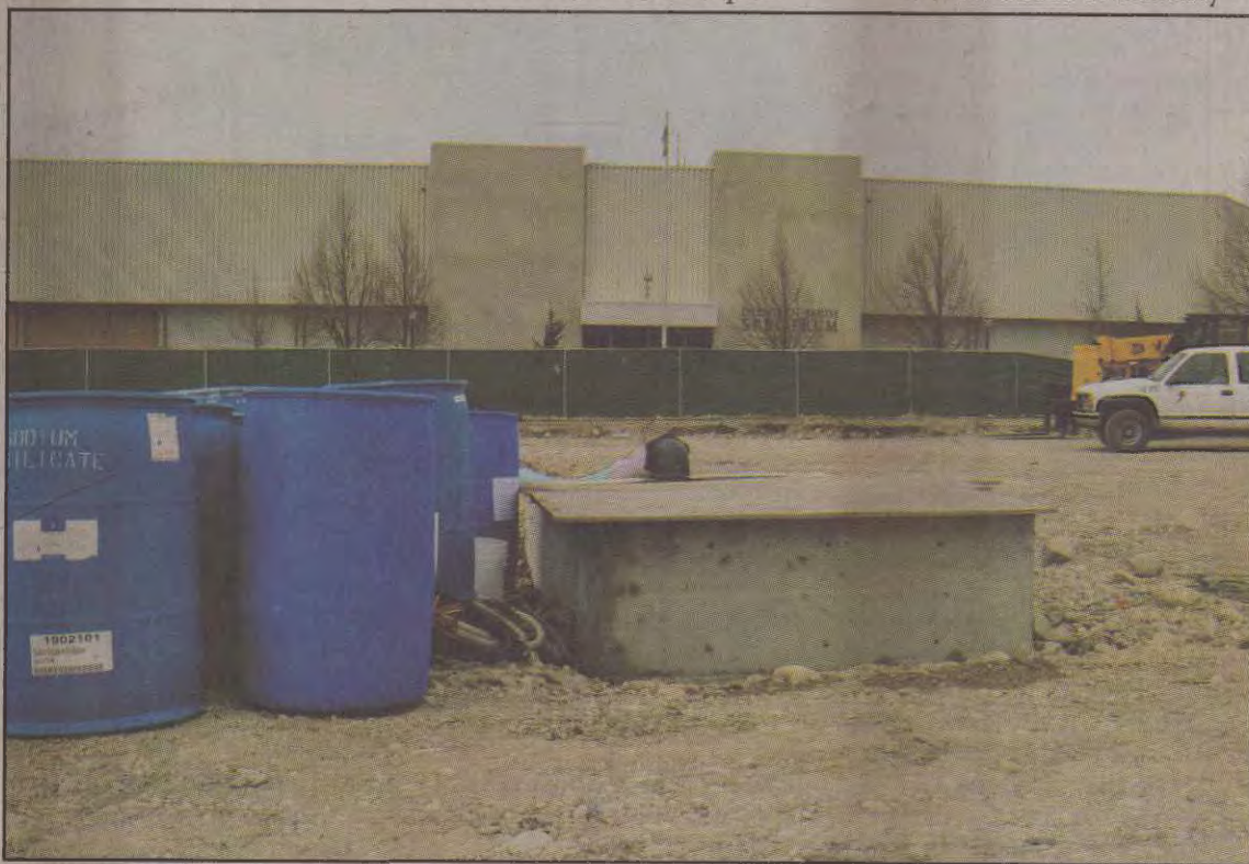
AFTER ALMOST A YEAR, construction of the thermal energy storage tank on the HPER Field is complete. Crews are currently filling the 2 million-gallon tank with water from a nearby fire hydrant. The tank will improve university air conditioning while saving energy and money. DELAYNE LOCKE photo
