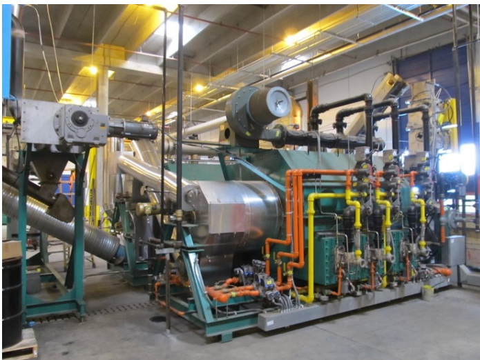
Figure 5. The Tucker RNG thermal conversion system uses forest biomass and other woody material as its fuel source Photo credit: Nate Anderson, USDA Forest Service
