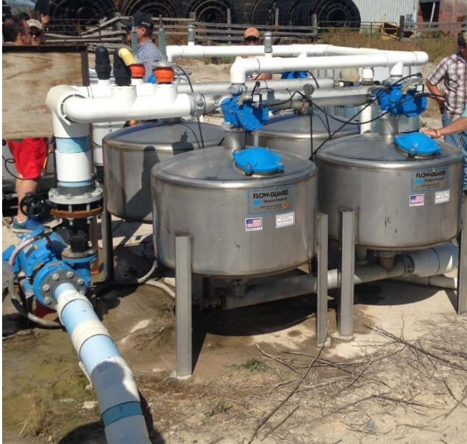
Figure 3. Media filters (four silver tanks).
