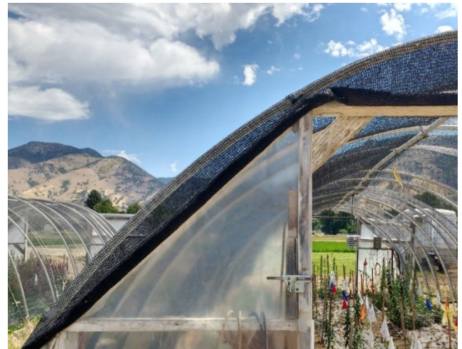
Figure 8. End of shade cloth wrapped around lath wood and attached to the high tunnel end-wall.
