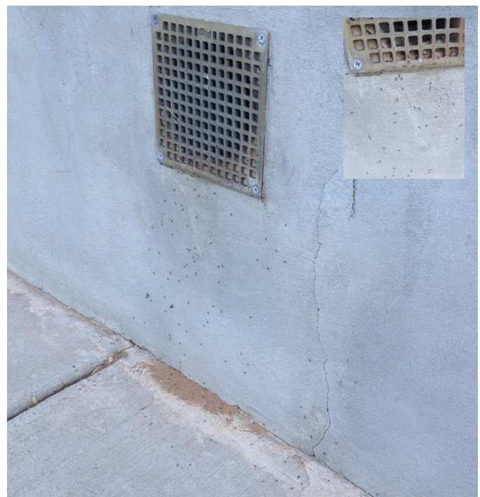
Fig. 8. Pavement ant workers accessing the interior of a building by crawling through a drain/foundation crack. Note the excavated dirt mound left by the pavement ants (Ryan Davis, Utah State University).
