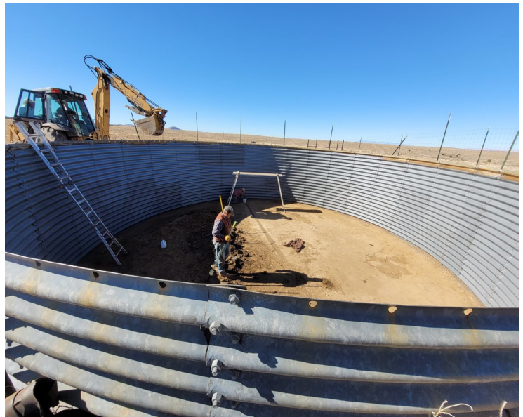
Figure 2. Steel Catchment Tanks Can Hold up to 200,000 Gallons of Water
