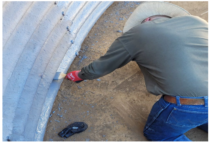
Figure 4. Completely Seal All Seams, Cracks, and Crevices
