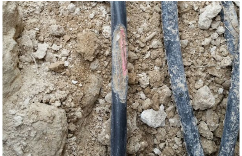
Figure 4. Damage to Buried Utility Lines by Pocket Gophers.
