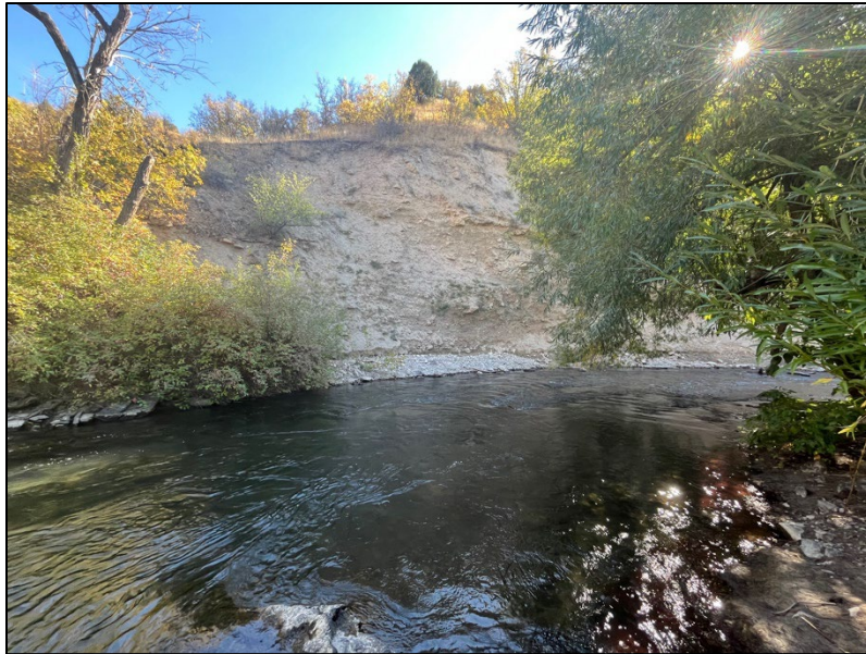
Figure 3. Steep, Eroded Riverbank Along the Logan River
