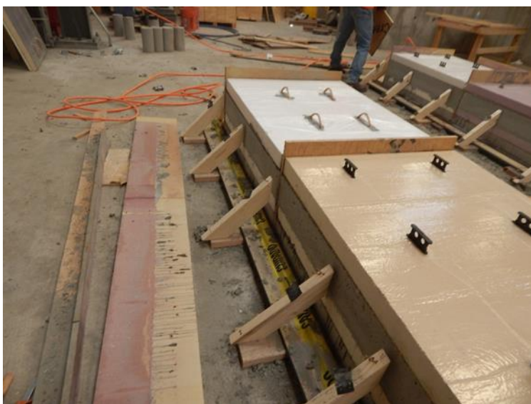
Figure 3-19 The highest set of forms is in place ready to pour the last concrete wythe
