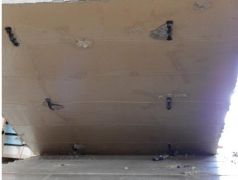
Figure 4-32 Shear fracture of Connector D (full specimen)
