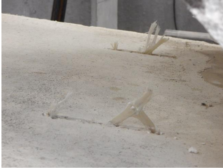
Figure 4-37 Tensile rupture of tension strut in truss.
