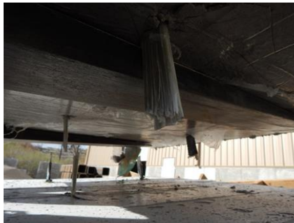
Figure 4-21 Dowel action failure of Connector B
