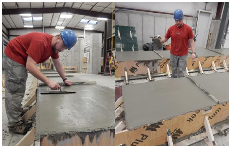
Figure 3-20 Taking special care to put a finished surface on the final wythe of the concrete
