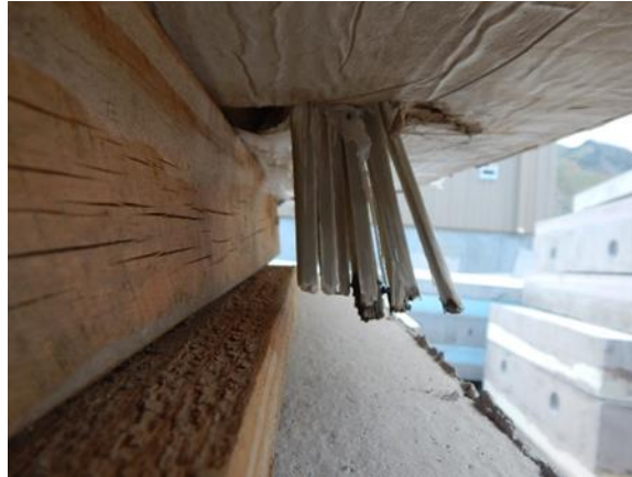
Figure 4-20 Dowel action causing delamination occurring along the width of Connector B
