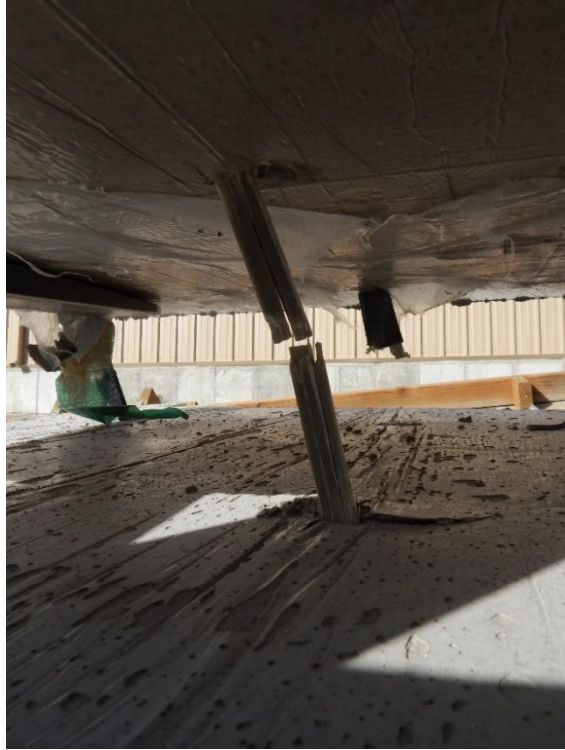
Figure 4-22 Dowel action occurring along the length of Connector B
