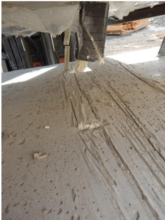
Figure 4-25 Shear fracture of Connector B
