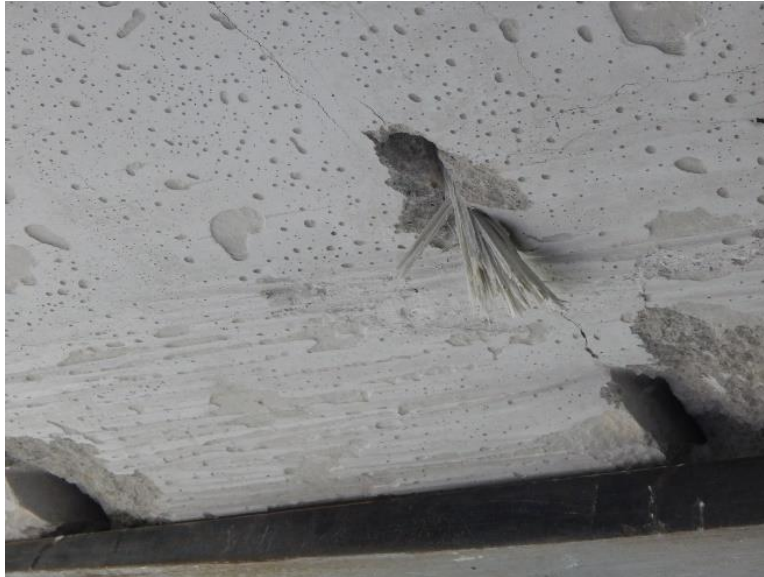
Figure 4-29 Shear fracture and dowel action of Connector C
