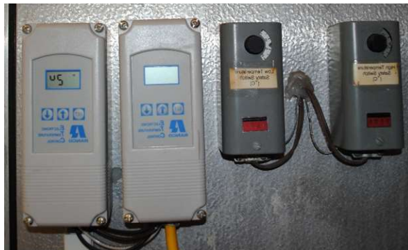
Fig. F.2.3. Separate day and night thermostats controlled each chamber.
