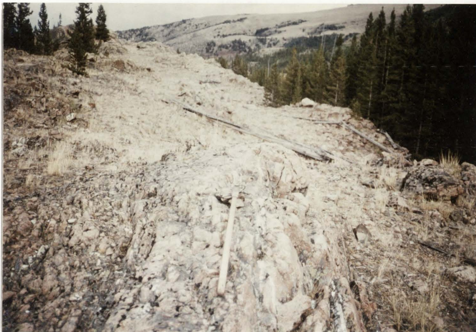
Figure 26. Photograph of outcrop at Gridpoint 5. View is approximately due east parallel to Jakey's Fork Fault. Walking stick lies on top of the densely fractured and veined outcrop. Most fractures and veins are nearly vertical, strike \approx east-west, and project through the offset Paleozoic rocks shown in Figure 29.
