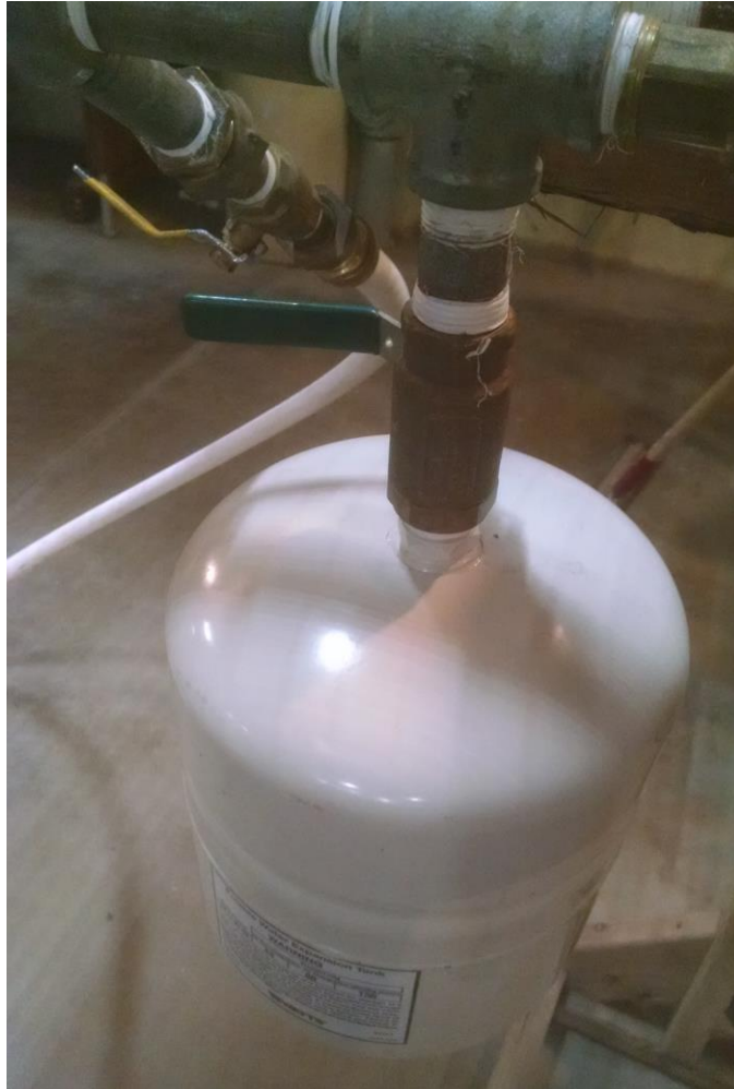
Figure 2. Thermal expansion tank included in test setup downstream of meters.
