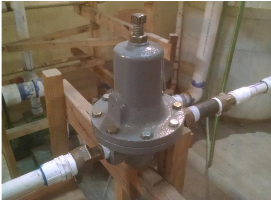
Figure 1. Pressure reducing valve placed upstream of test meters in laboratory setup.
