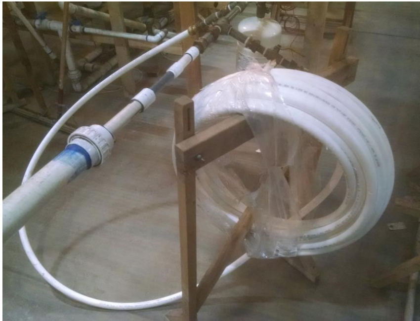
Figure 3. PEX tubing included in test setup downstream of thermal expansion tank.
