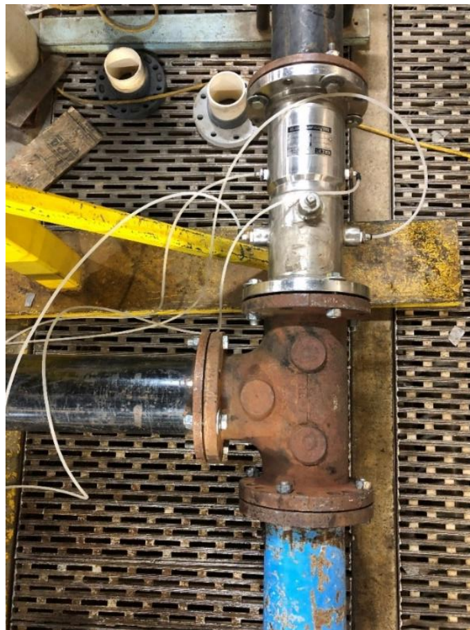
Figure 7. UVT with taps at positions 1 and 2 installed 0D on the through leg of a round cornered tee junction.
