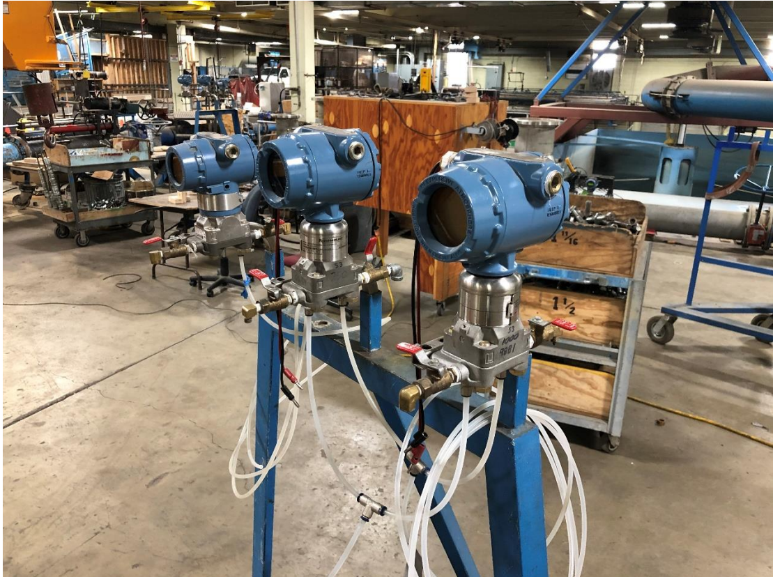
Figure 10. Pressure transmitters used to measure differential pressure.
